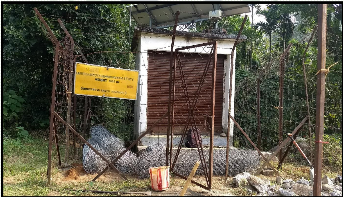
A Seismic station installed at College of Teacher Education, Rongkhon, Tura, Meghalaya with the financial assistances from MoES, Govt. of India.
